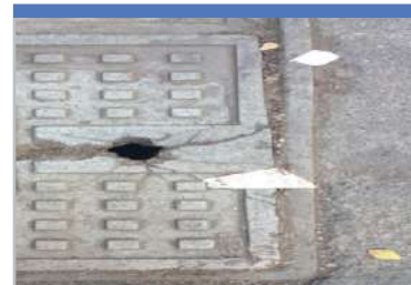
Condition of the Regular keyhole lifting arrangement of other make FRP manhole covers
